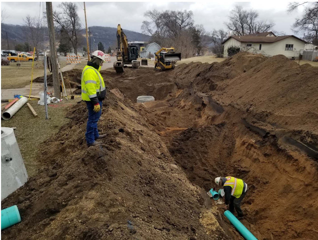
STH 35, Marquette Road Gerke Excavation Installing Sanitary Sewer Main Under Crawford Street
